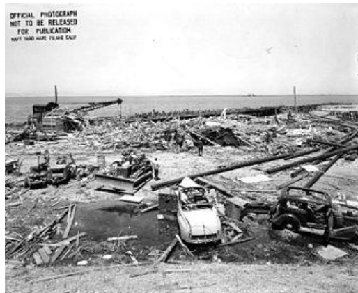
Photo # NH 96823 Damage at Port Chicago, Ca. View looking north toward pier. Cleaning up the damage at the remains of the pier.
